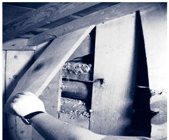
FIGURE 1. Rodent nesting material found inside the interior walls of a cabin — New Mexico, 2002
