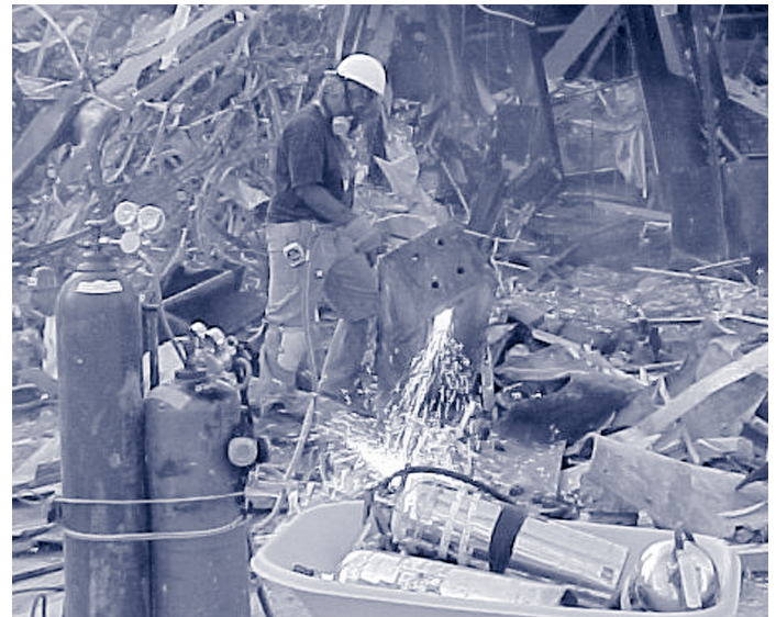
FIGURE 1. A worker clears rubble at the World Trade Center disaster site using an oxyacetylene torch
